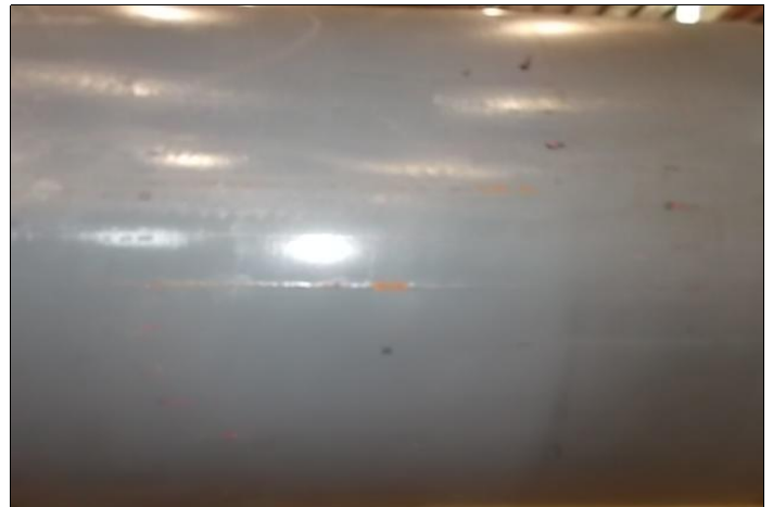
Bars are raising up in rotor. Minor core penetration
