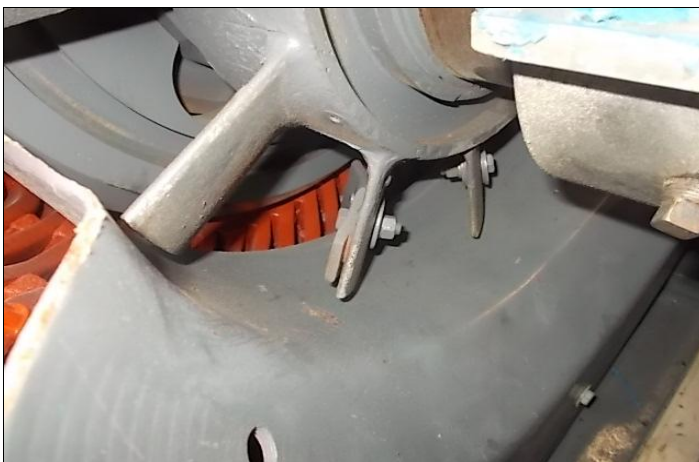
Excessive balance on internal fan blades
